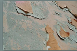
Peeling & Flaking of paint
