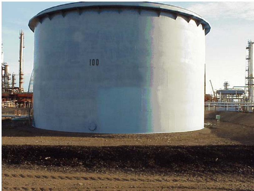
Picture 4: Crude oil storage tank at Esso Slagentangen in Norway coated in 1995 with a solvent-borne PU-topcoat. Light blue square at bottom of tank is a water-borne acrylic topcoat, coated at the same time as the PU-topcoat that has maintained its original color and gloss, while the solvent-borne PU-topcoat has faded.
