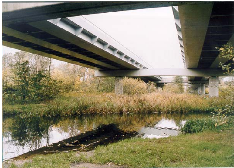
Picture 3: Thick water-borne coating system used for HD corrosion protection of load-bearing steel structures on a motor-way bridge
